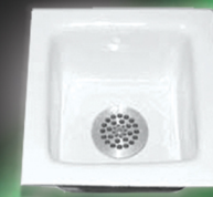
Floor Sink Drains
